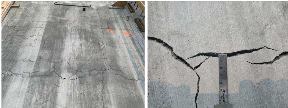
Figure 2. Significant Cracking at P13 Library Slab Pour
