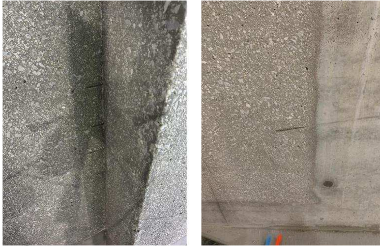
Figure 3. Partially Exposed Reinforcement at Architecturally Exposed Concrete Areas
